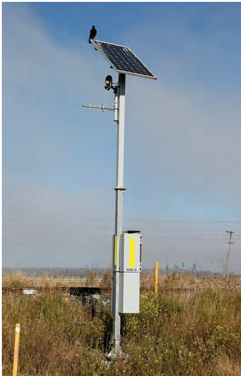
One of the two Train Detection Nodes (TDN) located on the approach to the Devon Park Road level crossing. The solar panel, radio antennae and equipment/battery cabinets can be seen in this view taken on 16 June. The TDN is activated by a Frauscher axle counter on the track.
